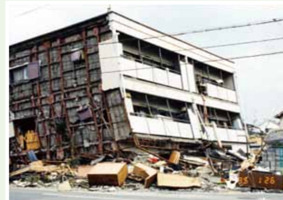
Gumuhong apartment. (Malaking lindol ng Hanshin, Enero, 1995)
